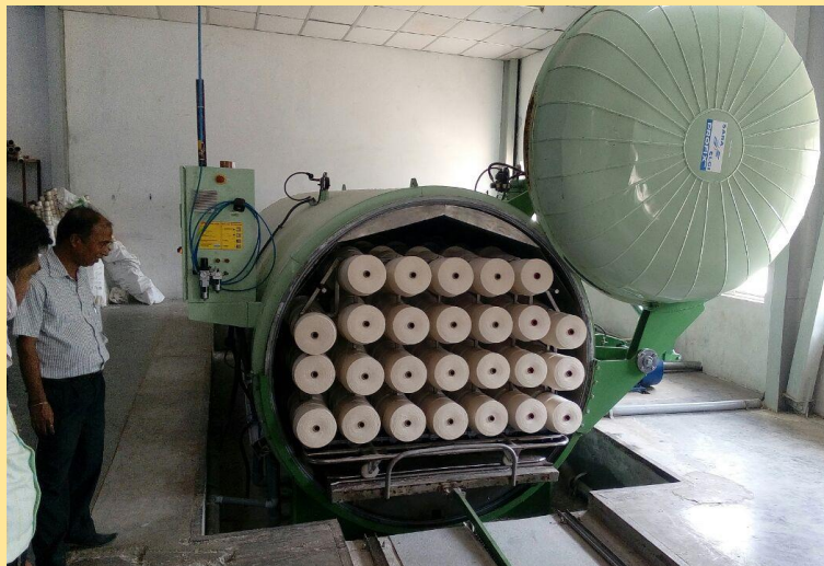
Turbine Section at Suryalakshmi Textile Pvt. Ltd.
